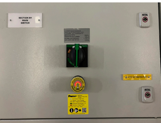
Additional Verisafe Absence of Voltage Tester in-situ
